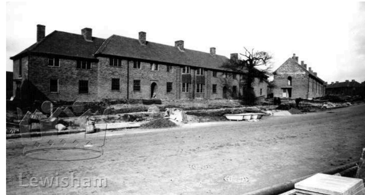
Ongoing construction work on the Bellingham Estate in 1923. The houses have been completed but baths are outside waiting to be plumbed in and the road is still unmade. Source: Borough Photos
