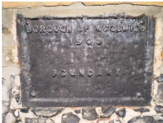
Boundary Marker (1903) on the east parapet of the bridge taking Weigall Road over the Quaggy
