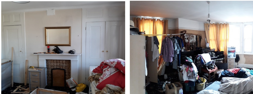
Figure 3.30 – Bedroom 10 (L) and 11 (R), each with chimney breasts which indicate that these rooms are part of the historic layout of the second floor.
