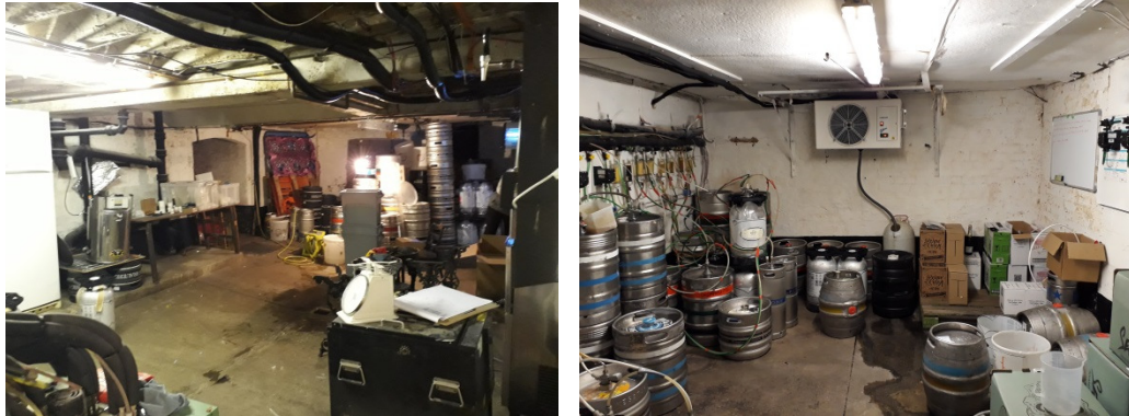
Figure 3.18 – The basement level of The White Hart is notably plain and utilitarian
