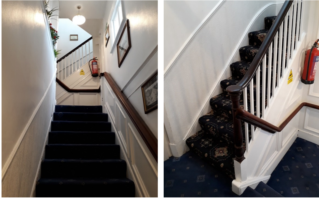
Figure 3.19 – Modern stair flight, leading to the original staircase, the lowest flights of which have been removed.
