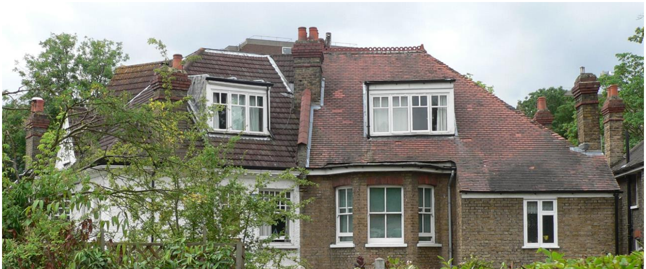
Image 56: Rear dormers of traditional form are fairly common. Front dormer windows are rare and generally not original or historic.
