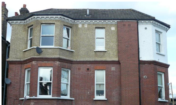
Image 78: Removal of chimney stacks can make a house appear truncated.
