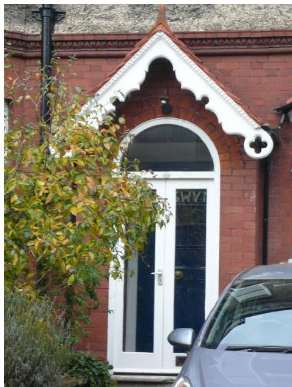
Image 75: infilling of porches hides the historic door, and is considered to be detrimental to the buildings character.
