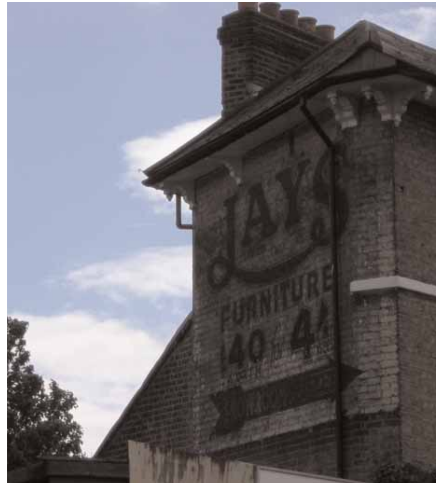
Detail on historic building on junction between Lee High Road and Gilmore Road
