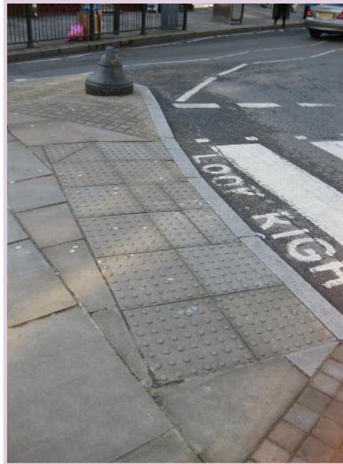
Dropped kerbs aid pedestrians in crossing the road, especially people with buggies and suitcases. They are essential for many wheelchair users.
