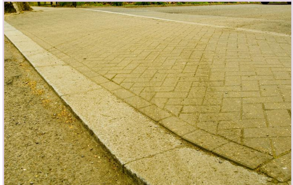
Footway crossovers allow vehicles to cross the footway to enter off-street parking or other developments.
