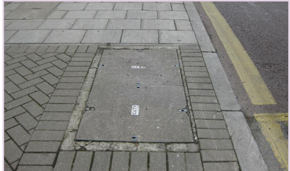
An inspection covers laid parallel to the kerb to minimise visual disruption of the footway
