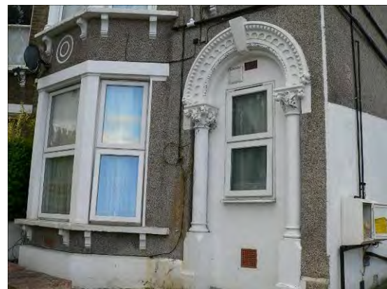
No. 220 Algernon Road (above) 82 Algernon Road (below): inappropriate alterations following conversion of the properties into flats.
