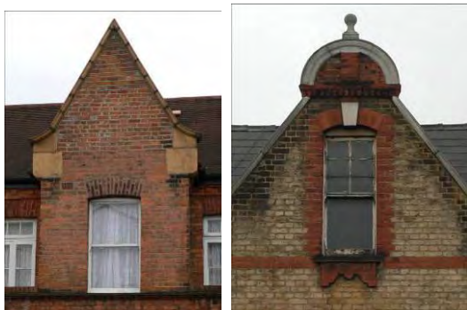
Above: Terracotta and brick details on gables in Algiers Road and at The Pavement.
