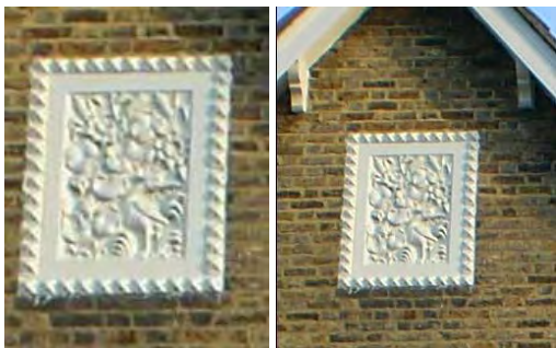
One of the foliage terracotta panels incorporated into the gables facing the street.
