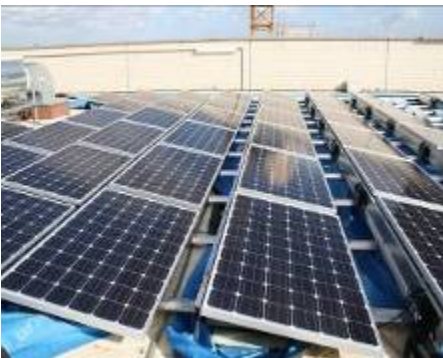
Solar Panels at Loampit Vale
