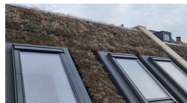
Photo 8: Good example of biodiverse living roof on sloping roof delivered on a new development in Lewisham
